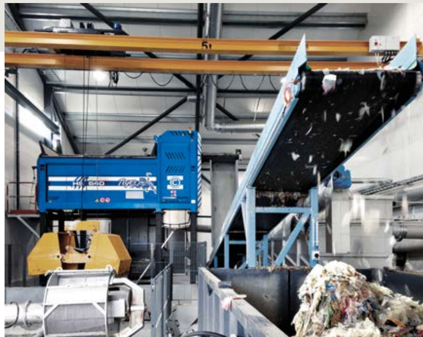
TIGER DEPACK HS 640 (FINLAND) / ORGANIC FRACTION OF URBAN SOLID WASTE FROM DIFFERENTIATED WASTE DISPOSAL
